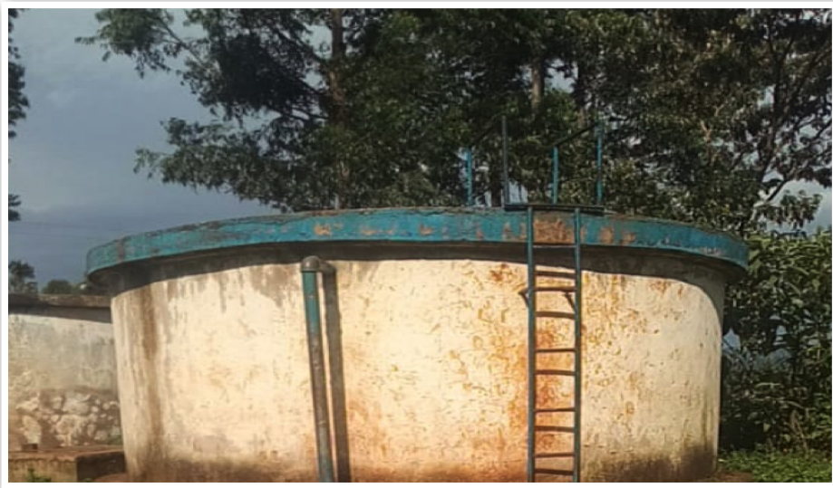
Figure 10: The Reservoir Tank for Cheribo Water Project
