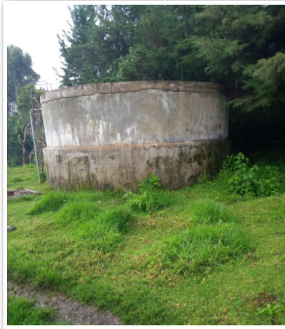
Figure 11: Chepseon Community Water Project Water Tank
