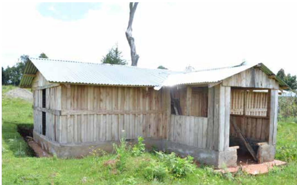
Figure 6: Stalled Tinet Dispensary Staff house as at November 2020
